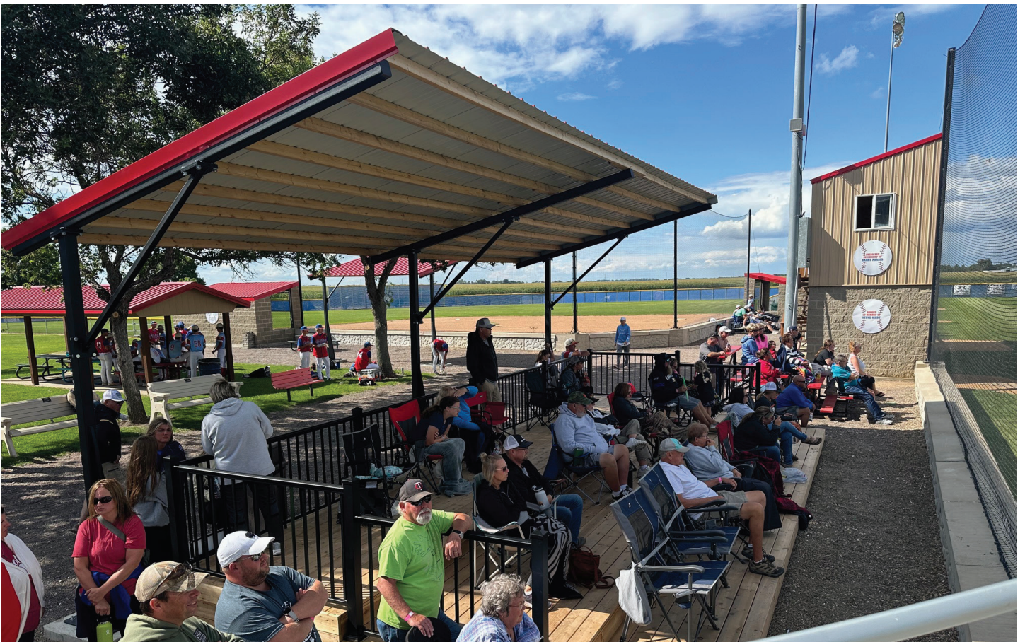
People were using the newly installed shelter on Locke-Karst Field. (Photo by Paul Kosel)
