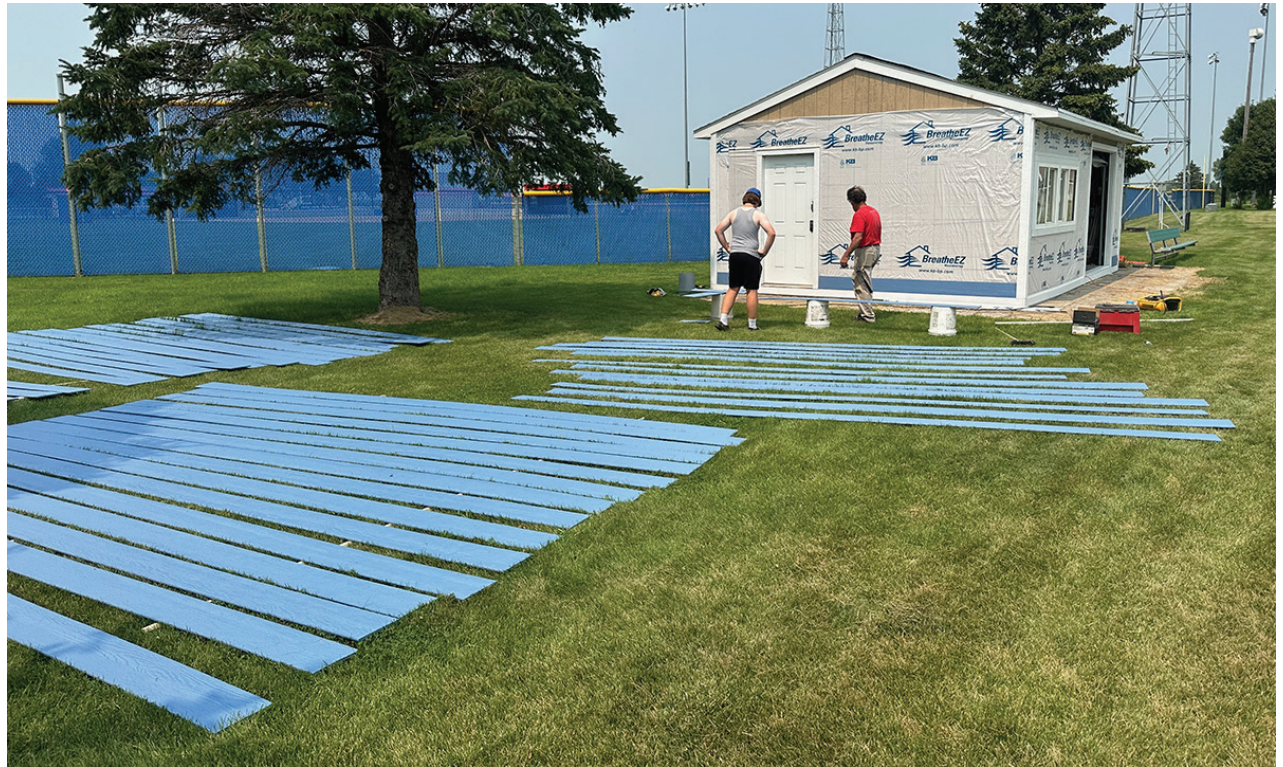
Jim Lane (right) and Nicholas Groeblichhoff were working on the soccer building. Several other city employees were helping on and off as Lane is redoing the outside of the building. The siding was all painted blue. (Photo by Paul Kosel)
