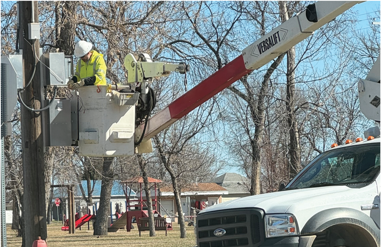
Paul Kosel, metering technician, busily works on the siren at the park on Wednesday morning. (Photo by Kellie Locke)
