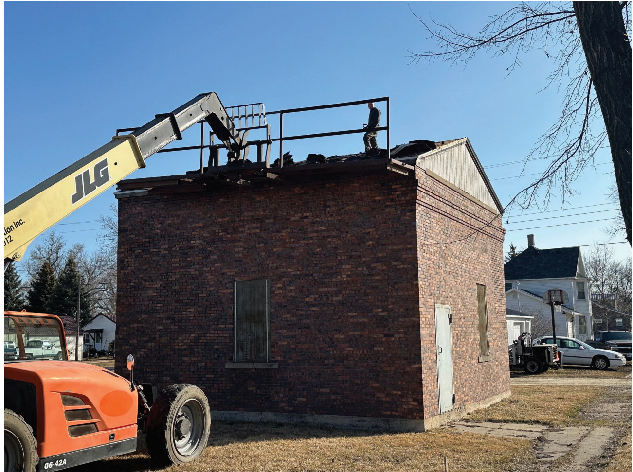
The roof historic jail building at the corner of N Third Street and East 1st Avenue was being worked on this past week. The building is now under ownership of the Groton Historical Society. (Photo by Paul Kosel)
