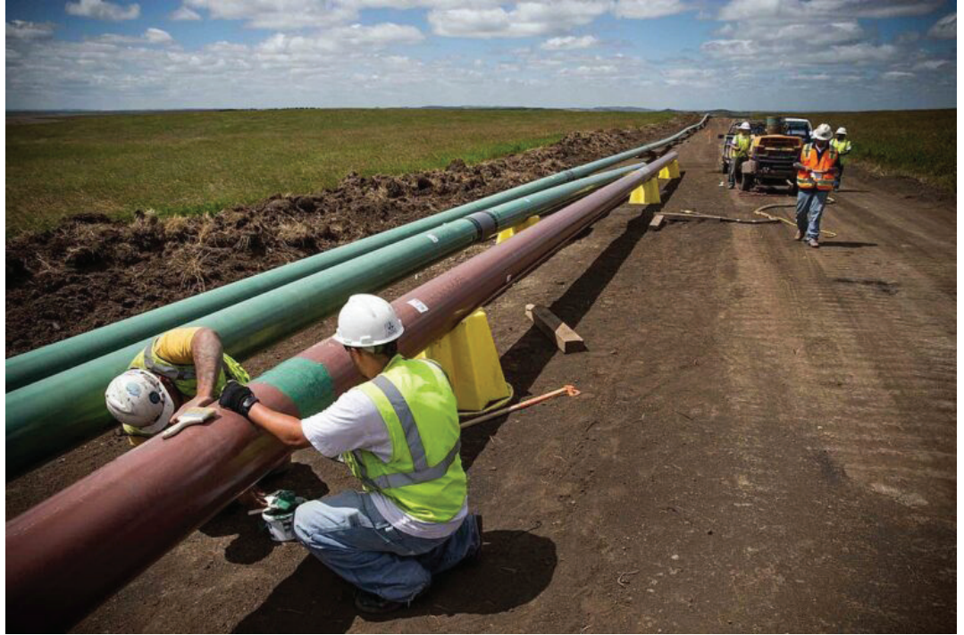
Construction workers specializing in pipe-laying work on a section of pipeline on July 25, 2013, outside Watford City, North Dakota. (An-
