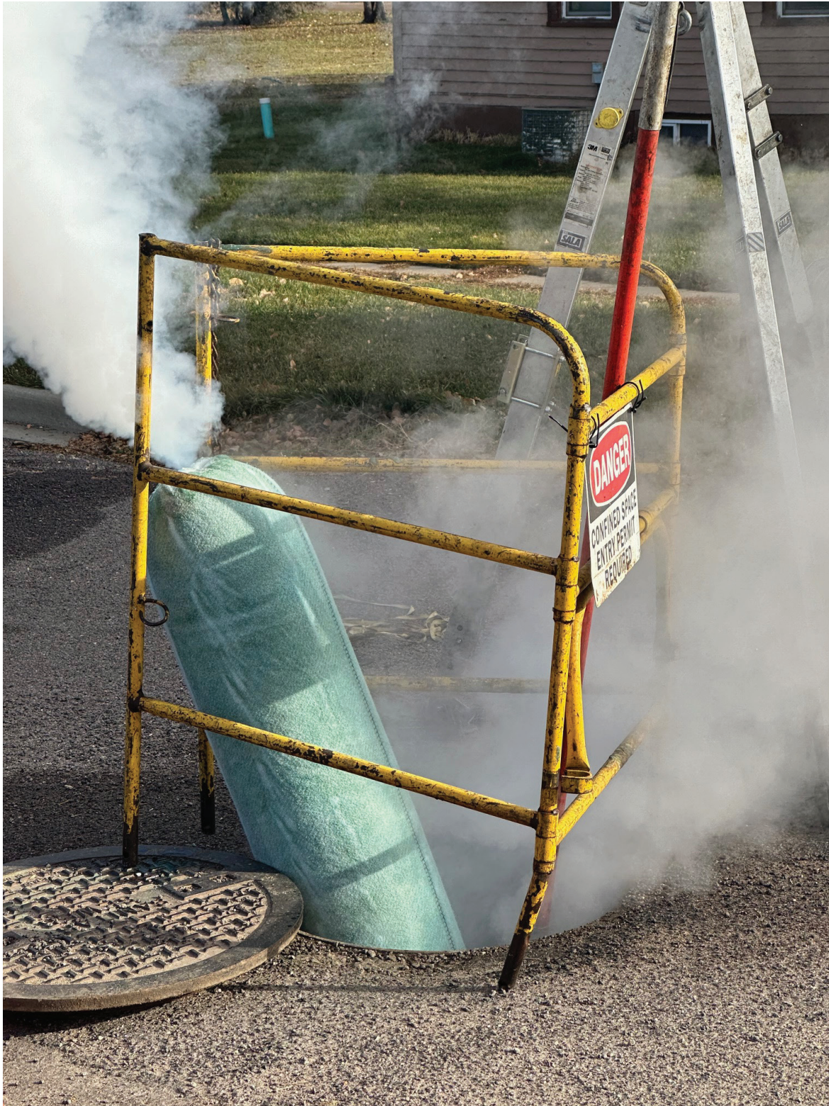
A section of the main sewer line between Railroad Avenue and Second Avenue is in the process of being relined. (Photo by Paul Kosel)
