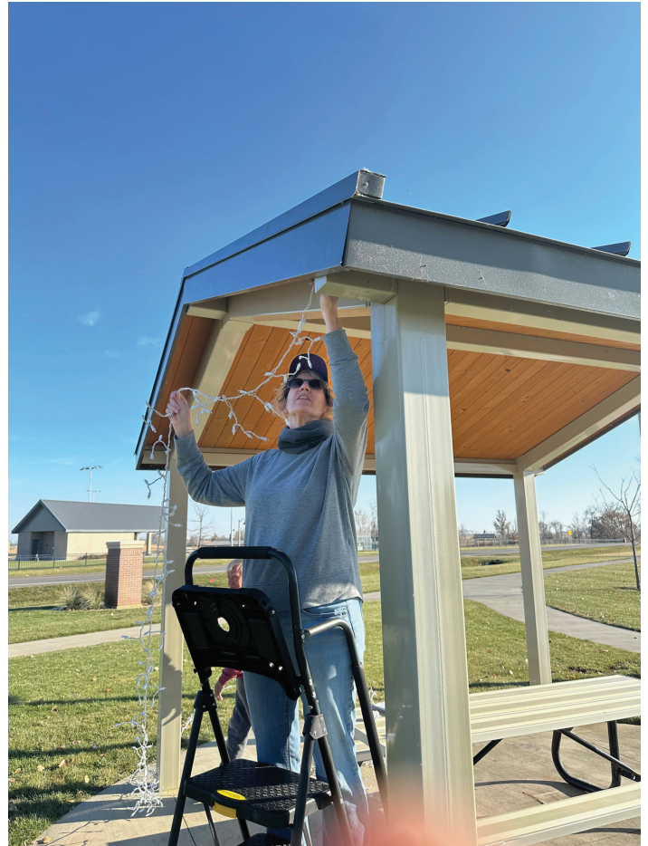
Julie Milbrandt Lillis started putting up the lights in one of the shelters. (Photo by Paul Kosel)
