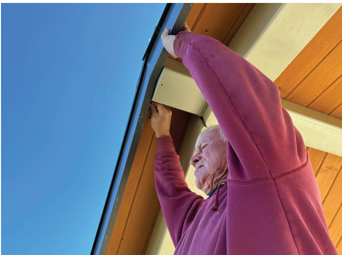
Larry Vietmeier is putting in hooks in the shelter for lights. (Photo by Paul Kosel)
