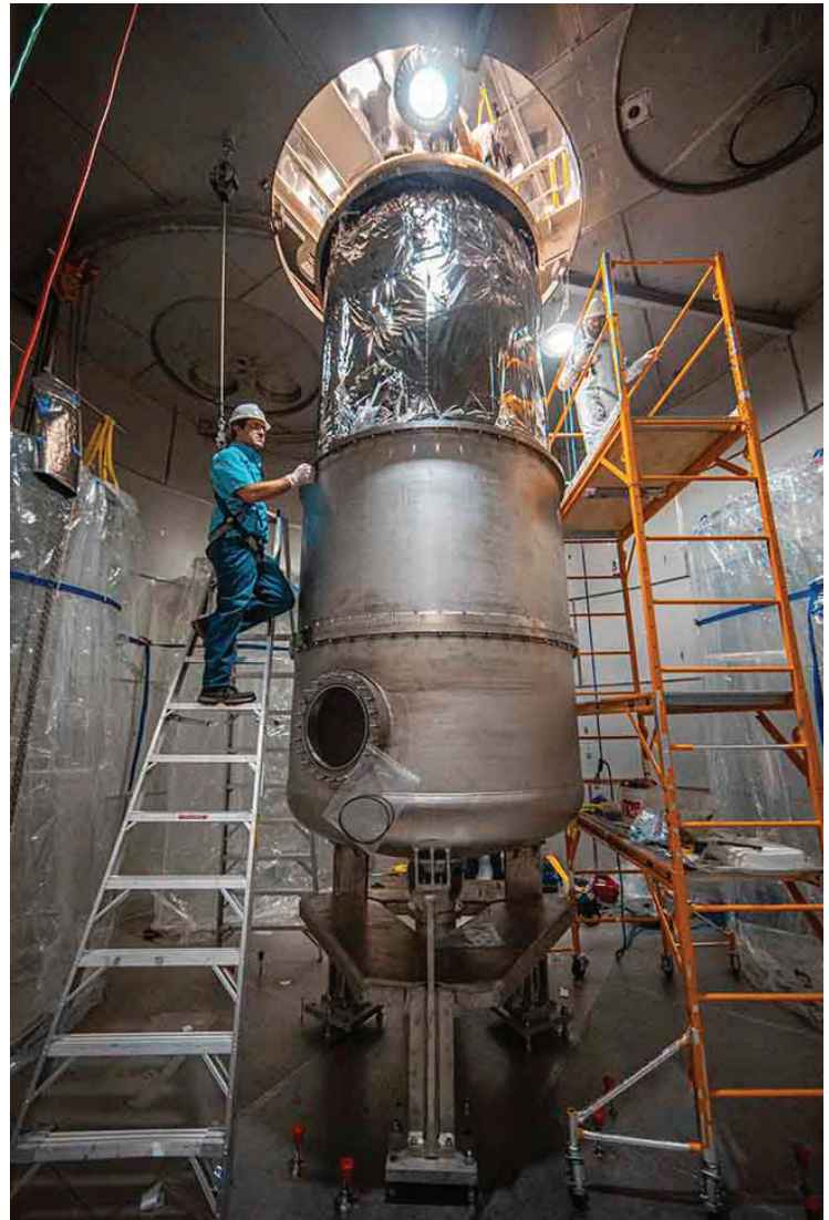
Engineers, Charles Maupin (left) and Jake Davis work to install one of the LUX-ZEPLIN (LZ) chambers in 2019. LZ is a next-generation dark matter experiment in South Dakota. Photo credit: Nick
