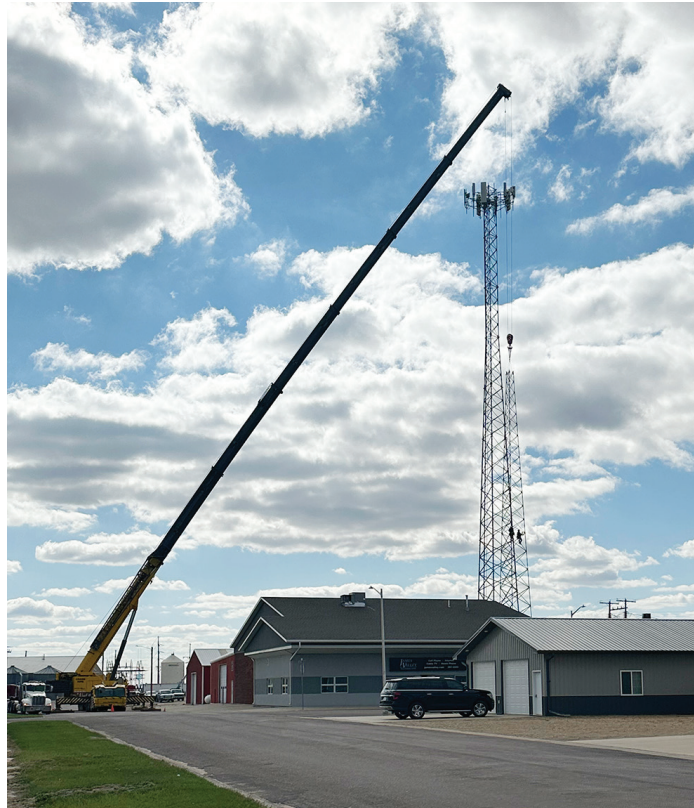
The smaller tower at James Valley Telecommunications was taken down in pieces on Monday. (Photo by Paul Kosel)
