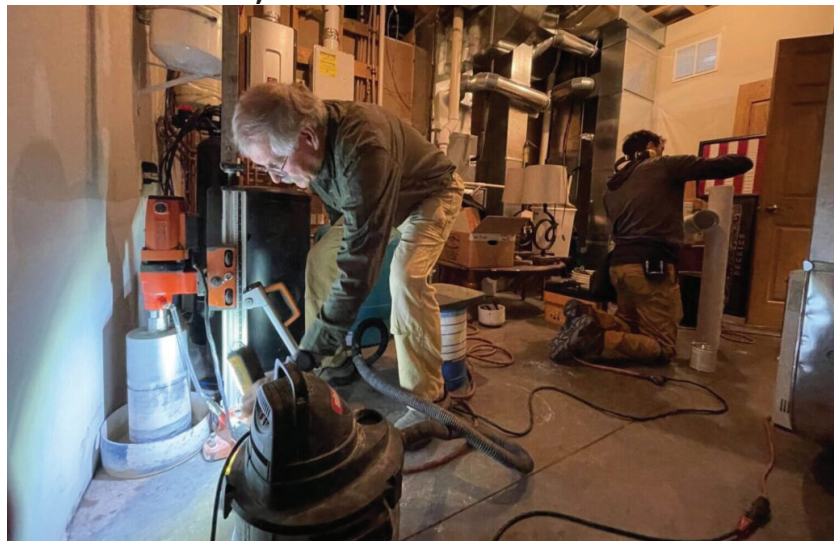
Bob Burns and his son Murray LaHood-Burns, of Earthorizons Inc., install a radon mitigation system in a Rapid City home on March 24, 2023. (Seth Tupper/South
