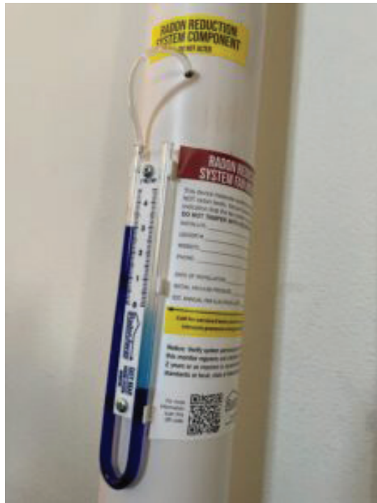
Part of a radon mitigation system in a Rapid City home. (Seth Tupper/South Dakota Searchlight)
