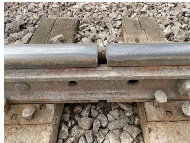
A significant gap can be seen between two sections of a rail line that runs east-west through downtown Rapid City. Many rail lines in South Dakota have been in operation for a century or more and require frequent maintenance. Photo: Bart Pfankuch, South Dakota News Watch
