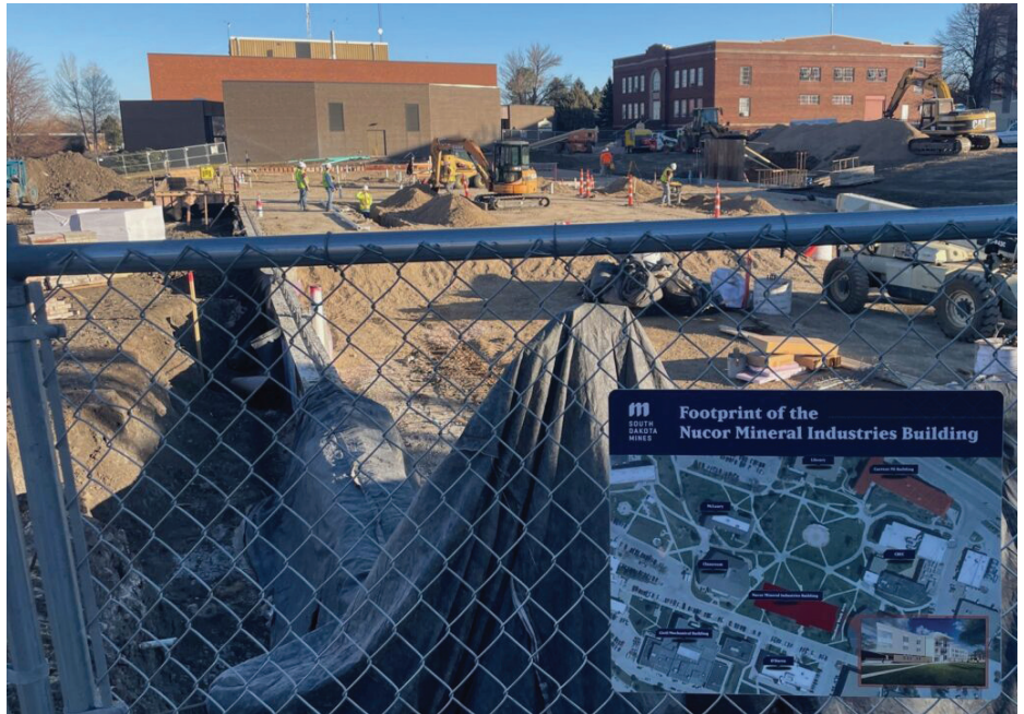
To save money, the minerals lab now under construction on the campus of South Dakota Mines in Rapid City was moved to a flatter, more centralized location. The relocation saved about $4 million in project costs. Photo: Bart Pfankuch,
