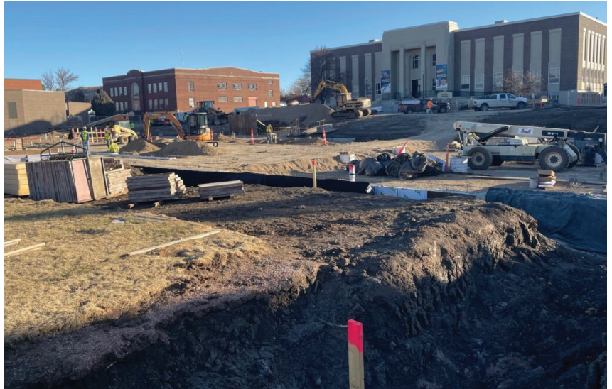
High inflation and labor costs have driven up the cost of several projects approved by the South Dakota Board of Regents, including the minerals lab now under construction at South Dakota Mines. Photo: Bart Pfankuch, South Dakota News Watch
