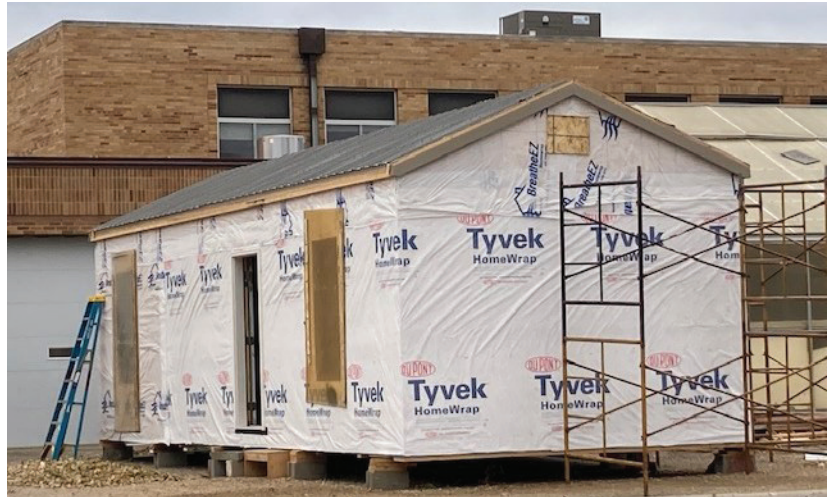
This is the exterior view of tiny House under construction by the Groton Area shop students. (Photo by
