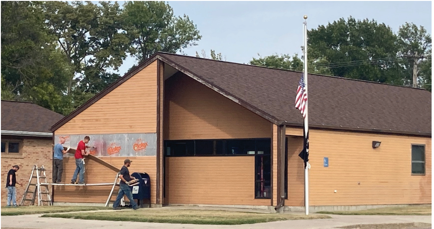
The Groton Post Office is getting a new facelift as the siding started coming off on Wednesday.
