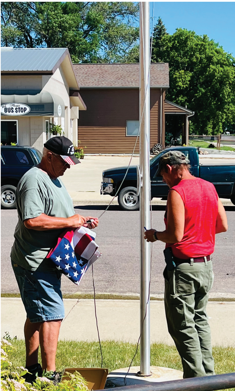
Doug Hamilton and Paul Kosel finish putting the hardware on the rope on the new flag pole at City Hall. (Photo by April Abeln)
