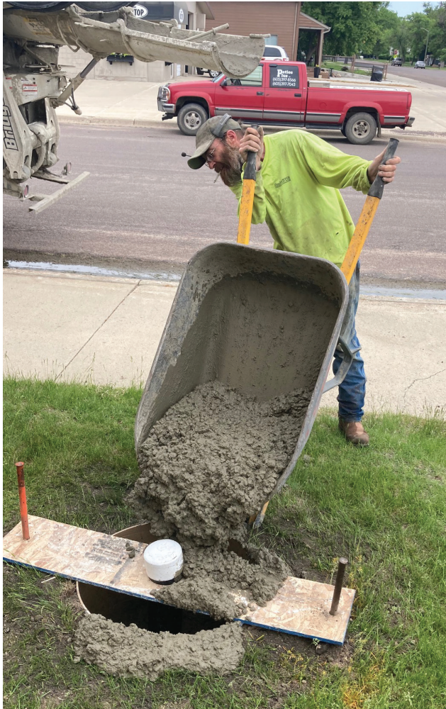
Flag Pole Base Poured Joe Foertsch of Patios Plus is pouring the concrete into the hole in front of City Hall. This will be the site for the new flag pole.
