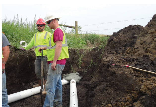
Peggy Hoogestraat said that drain tiles in her farm field west of Hartford were damaged during construction of the Dakota Access Pipeline, and that she hired her own construction workers to oversee the repairs done by workers with DAPL.
