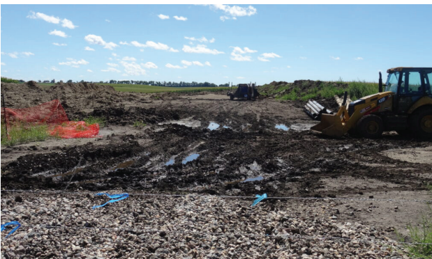
Ruts and depressions in the land, such as these and sometimes worse, occasionally result along the Dakota Access Pipeline route that runs through Peggy Hoogestraat's land in western Minnehaha County. The ruts can make farming difficult and cause damage to the legs and feet of cattle. Photo: Courtesy Peggy Hoogestraat
