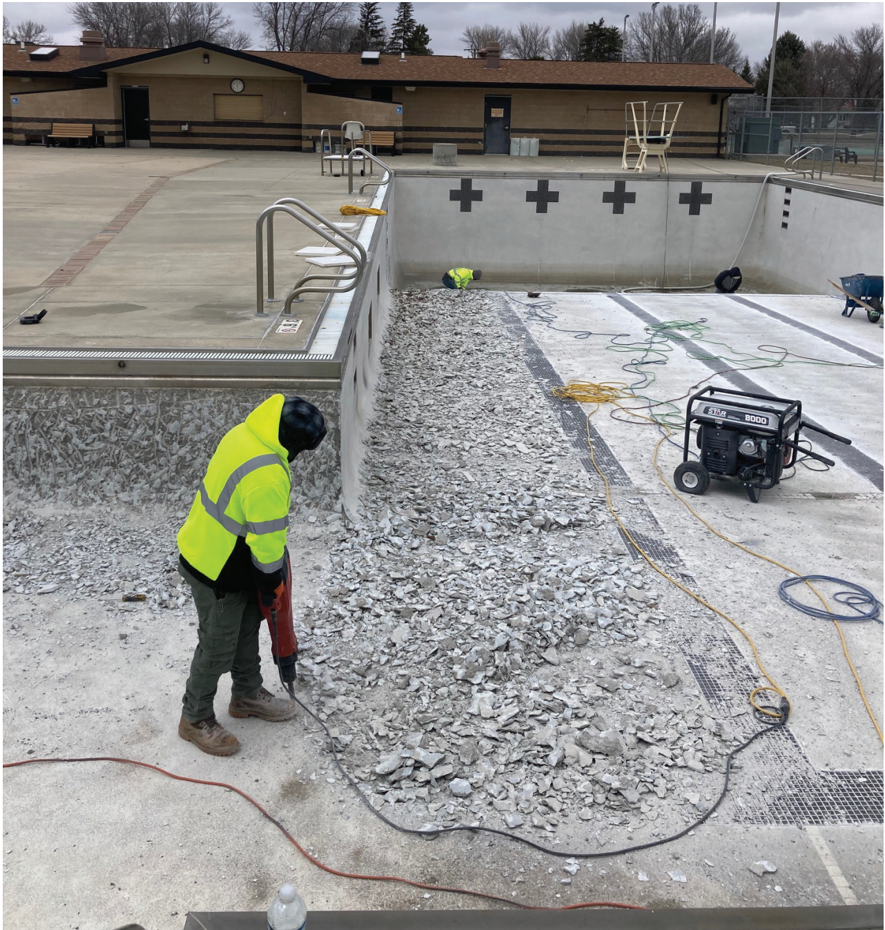
The demolition of the Groton pool has begun. The plaster will be removed and replaced later this month. (Photo by Paul Kosel)
