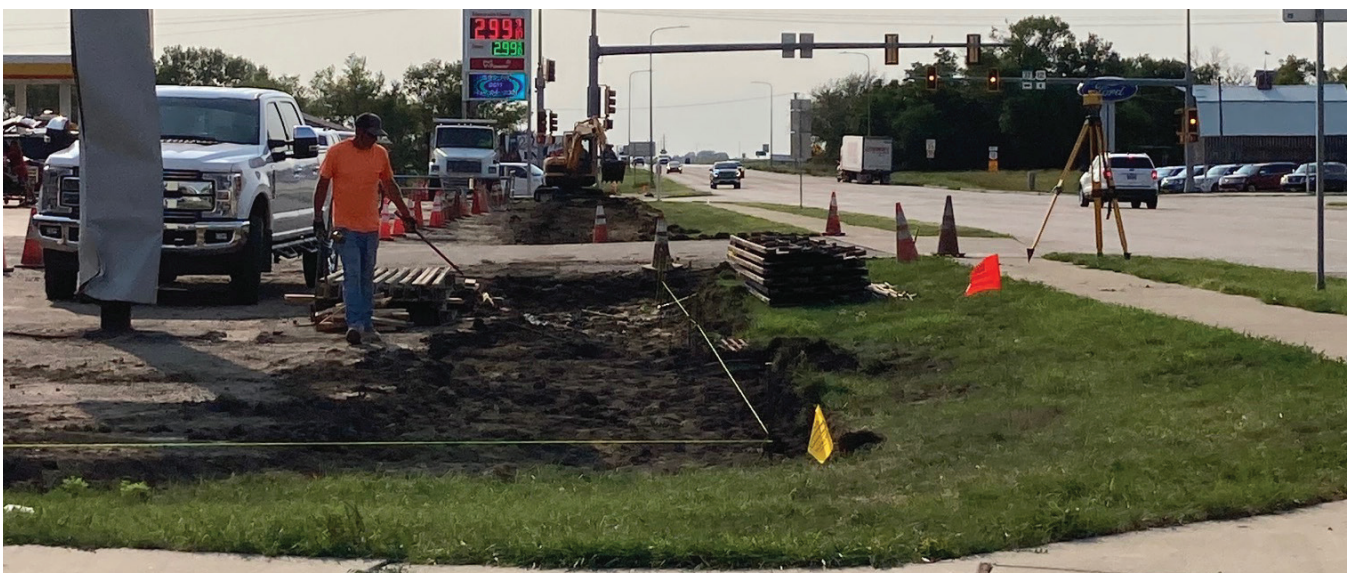
The minimall and Ken's Food Fair are having a new curb installed on the north side of the parking lot. (Photo by Paul Kosel)
