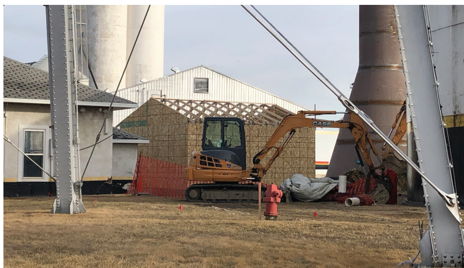
Work started Monday on the new structure going up for the new pump house.
