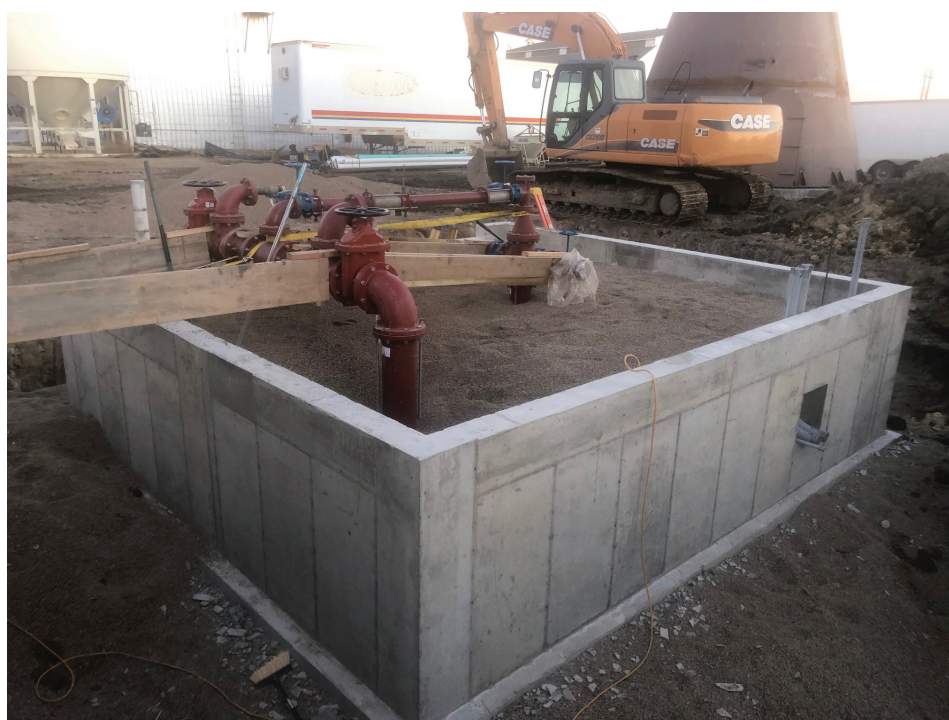
Work is starting to resume on the Groton Water Tower project. The above shows the footing for the new building that will be put up, just south of the existing pump room.
