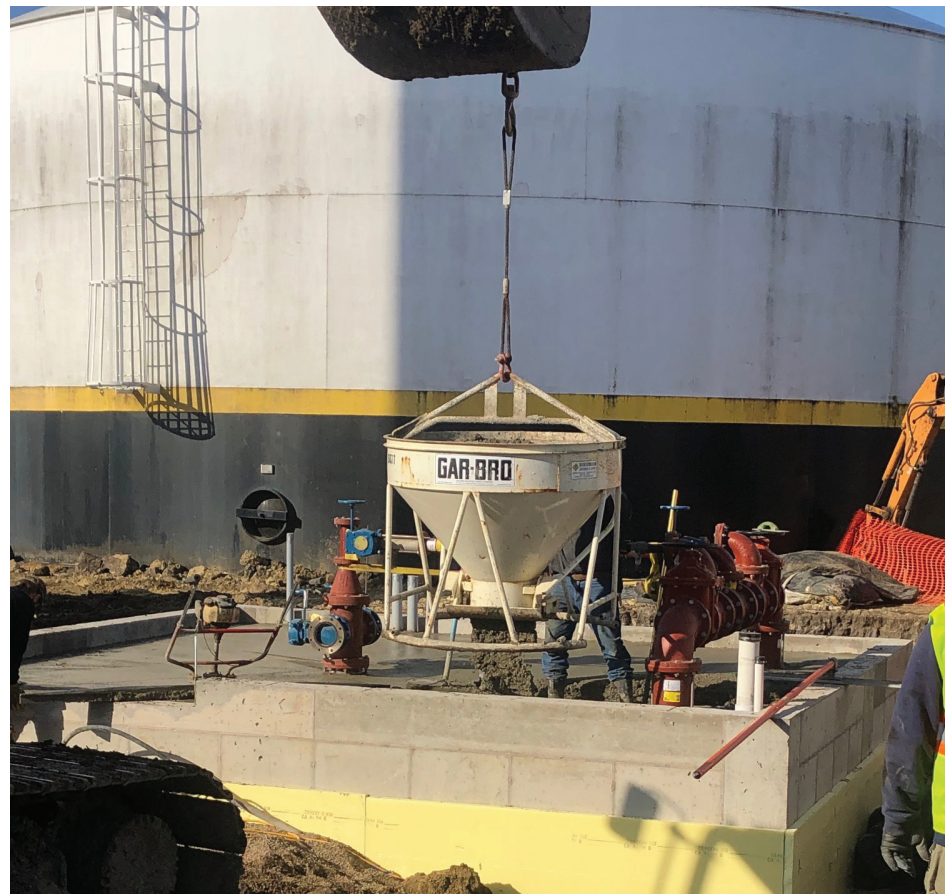
Concrete was lowered down in this carrying device and then released. The floor for the new pump room was poured on Thursday. (Photo by Paul Kosel)
