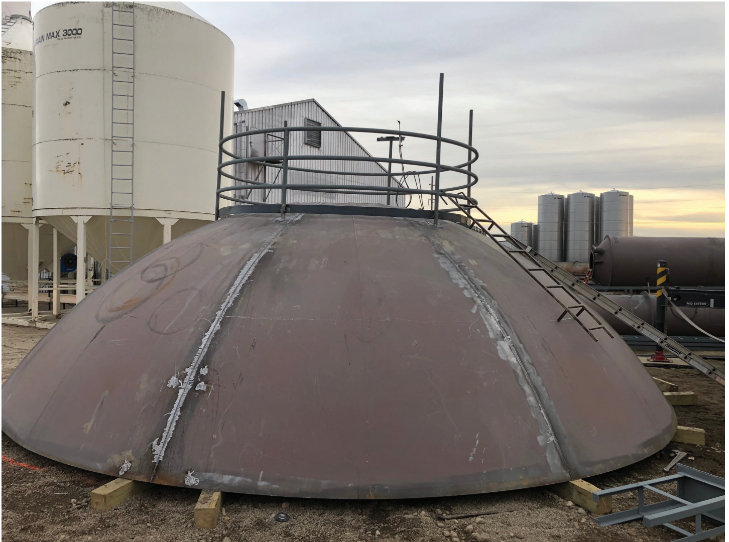
The ladder and the safety railing was attached to the roof of the water tower on Wednesday. (Photo by Paul Kosel)
