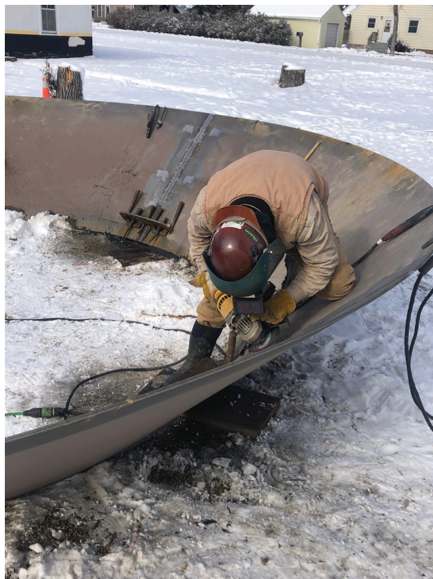
Welding and grinding. And more welding and grinding and work continued a week ago on Sunday on the new Groton water tower. (Photos by Paul Kosel)
