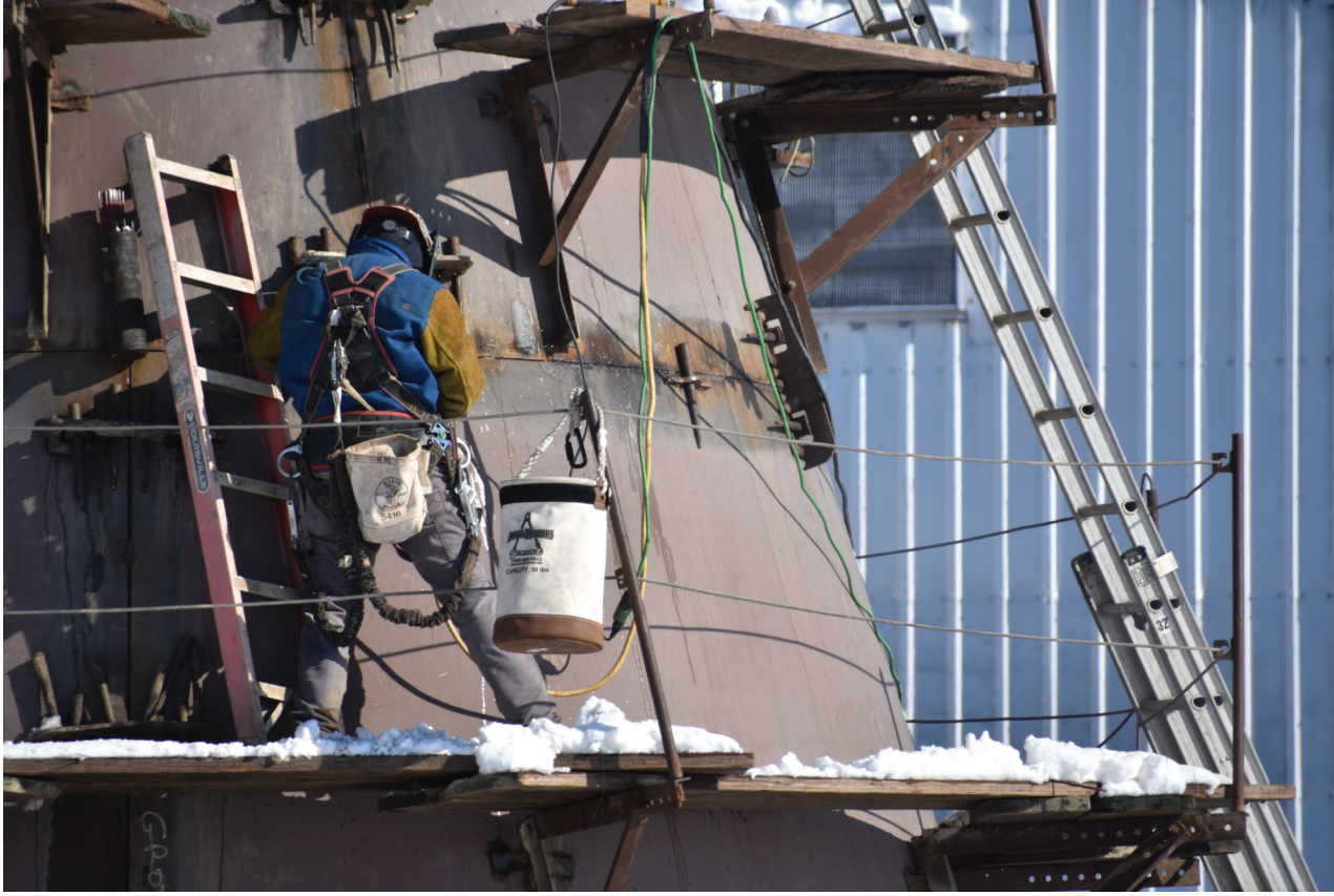
There is a lot of equipment being used as the scaffolding is attached to the tower while the welders weld the new water tower together. (Photo by Paul Kosel)
