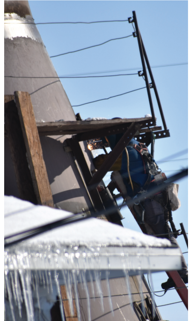
You can see the ball of fire as welding work is being done on the new water tower. (Photo by Paul Kosel)
