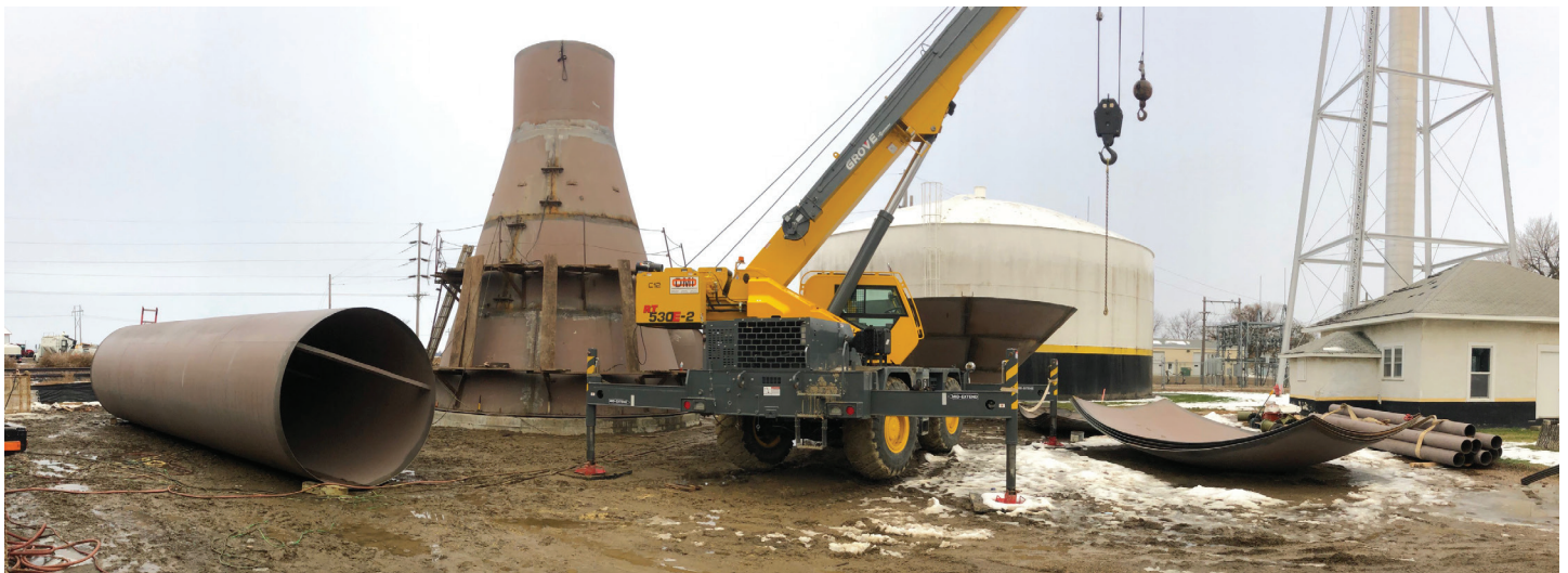
Another section to the water tower was delivered on Thursday. The main column is pictured on the left. Also dropped off was the pipe for water delivery that will be installed inside the column. That bundle is located to the right in the photo. (Photo by Paul Kosel)
