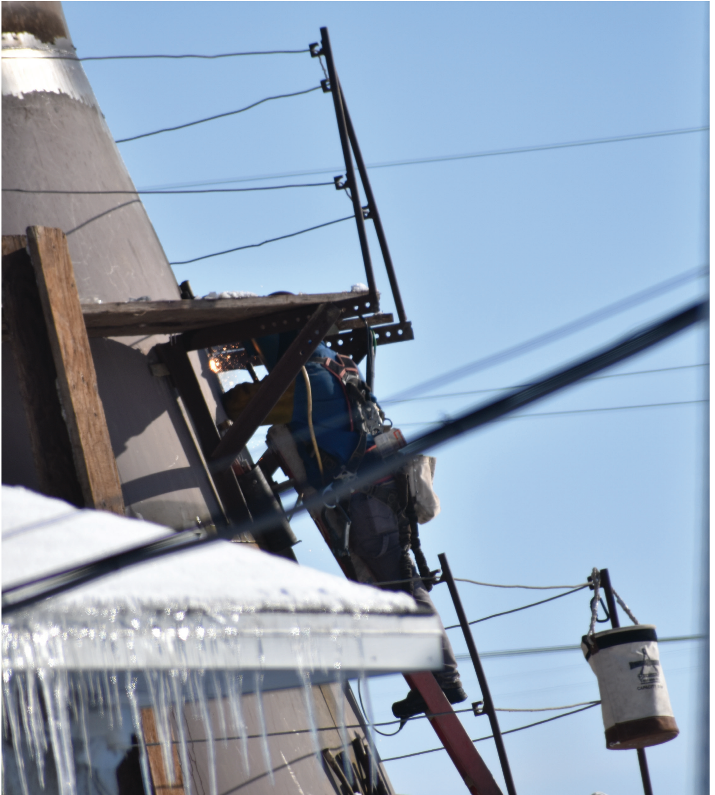
You can see the ball of fire as welding work is being done on the new water tower. (Photo by Paul Kosel)
