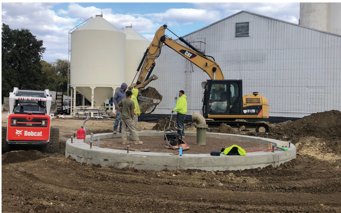
The finishing touches are being applied to the base of the new water tower. (Photo by Paul Kosel)
