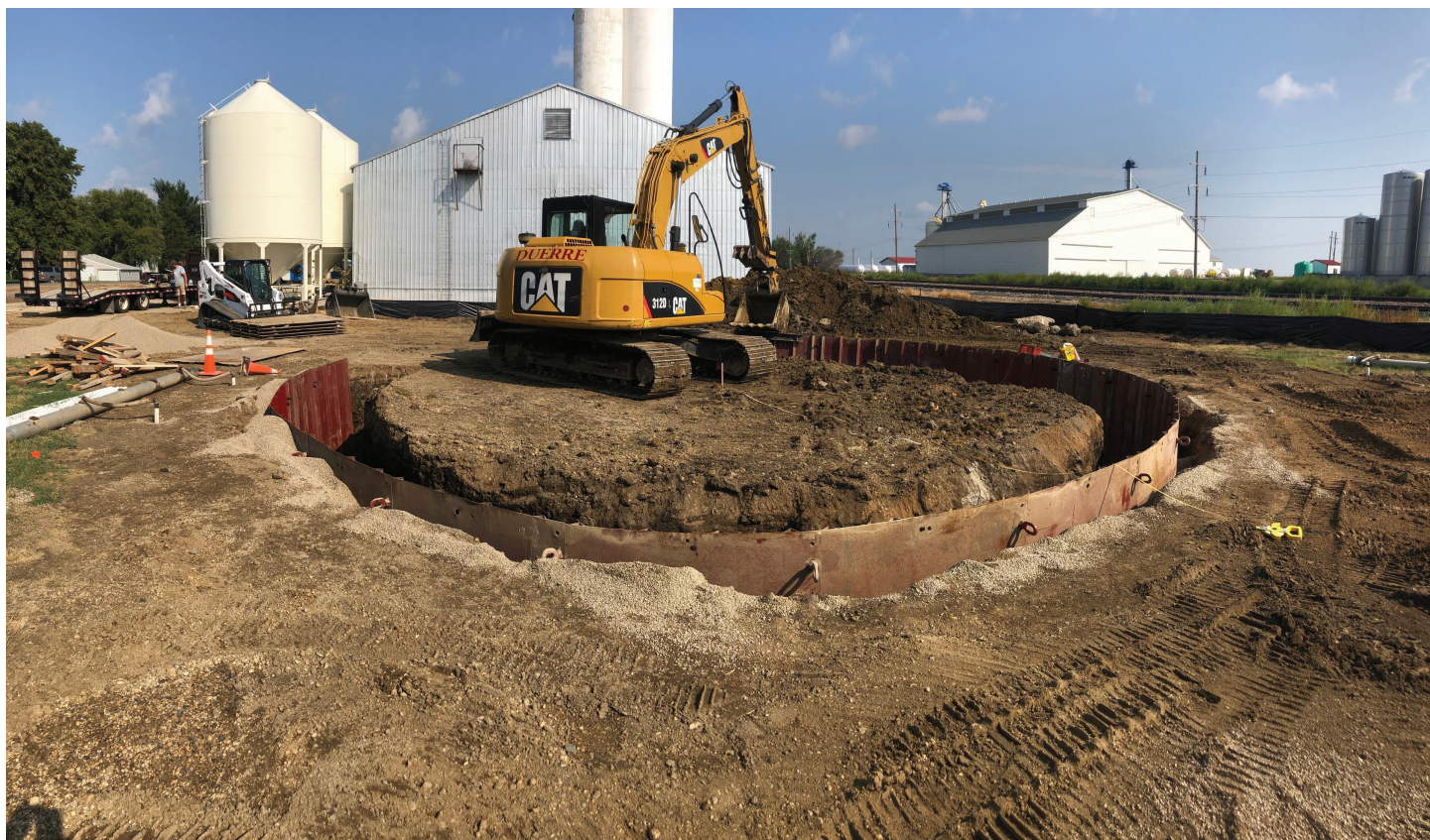
The hole is being dug for the footing for the new water tower. (Photo by Paul Kosel)
