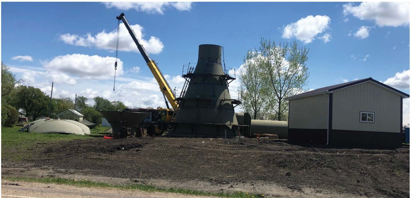
Work is well underway for the new Langford water tower. (Photo by Paul Kosel)
