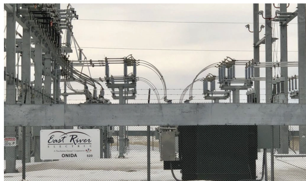
East River Electric Cooperative serves as the electricity transmission co-op for eastern South Dakota and built this substation near Onida to serve the Ringneck Energy ethanol plant recently built in the city. Electric co-ops such as East River Electric have been trying to change state law in recent years to restrict the ability of municipal utilities to take service territory from co-ops. Photo: Nick Lowrey, South Dakota News Watch
