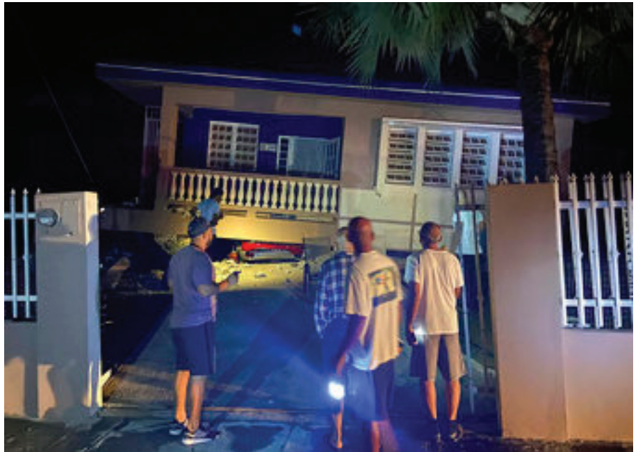
A collapsed building with car crushed underneath, following an earthquake in Yauco, Puerto Rico, Tuesday Jan. 7, 2020. All the occupants of the home are reported to be uninjured. A 6.5-magnitude earthquake struck Puerto Rico, the largest in a series of quakes in recent days, and caused heavy damage in some areas. (J. Miguel Santiago Twitter via AP)
