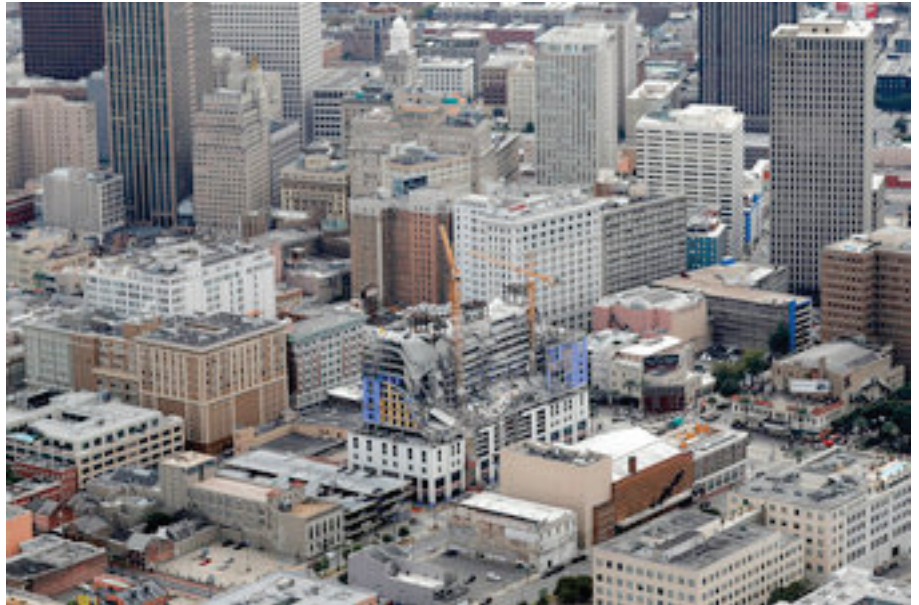
This aerial photo shows the Hard Rock Hotel, which was under construction, after a fatal partial collapse in New Orleans, Saturday, Oct. 12, 2019. (AP Photo/Gerald Herbert)
