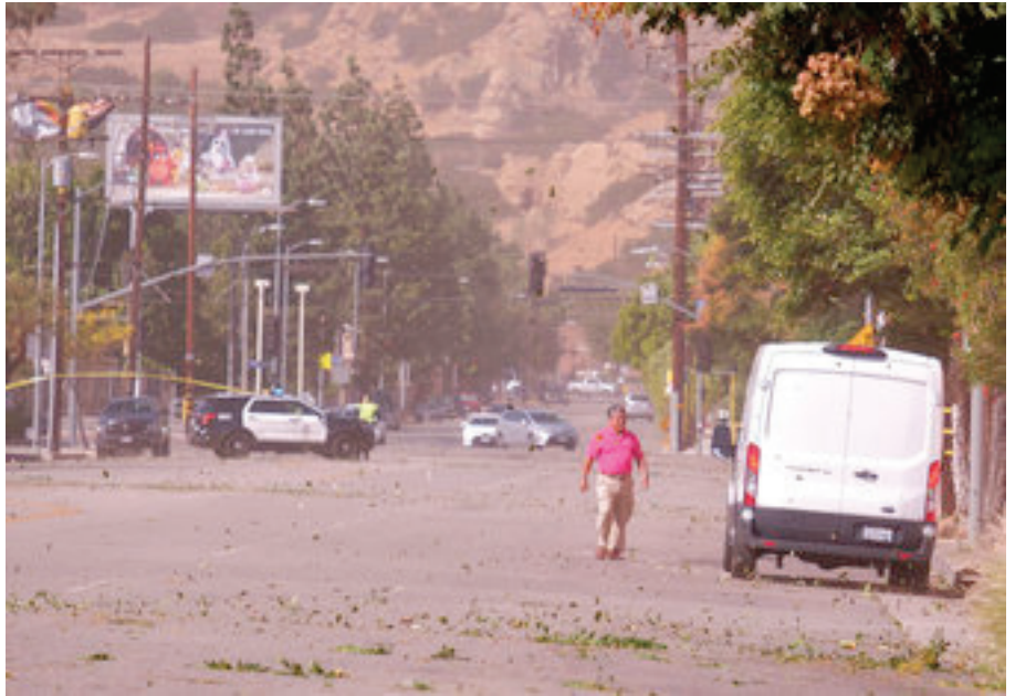
Strong Santa Ana winds in Chatsworth, Calif., blew across power lines causing them to arc and transformers to explode. Power was out for street signs, businesses and residents along Devonshire St. from Topanga Canyon Blvd. to Variel Ave. on Thursday, Oct. 10, 2019. (Dean Musgrove/
