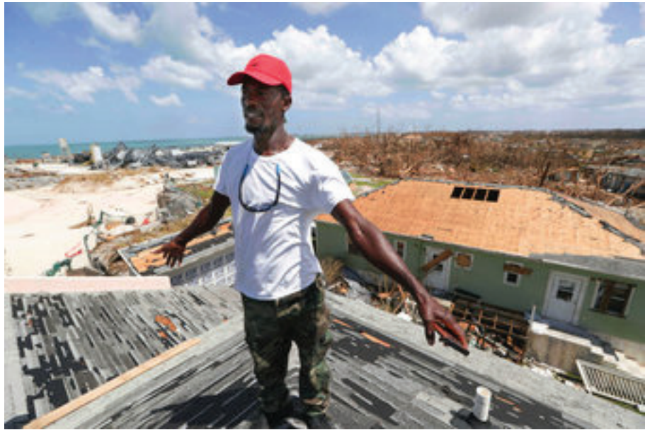
Jackson Blatch starts repairs on the roof of his home in Marsh Harbor, Abaco Island, Bahamas, Saturday, Sept. 7, 2019 after Hurricane Dorian hit. (AP Photo/Fernando Llano)
