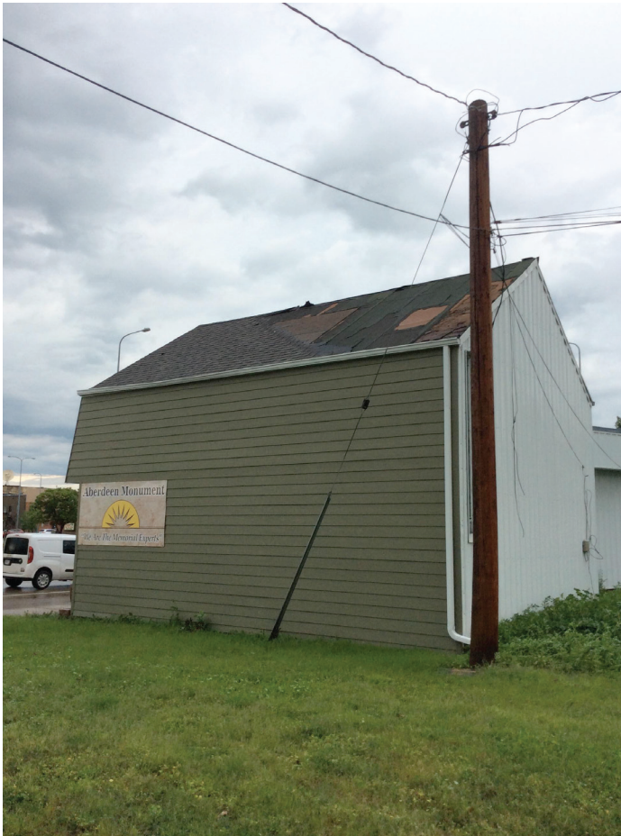
Shingle Damage in Aberdeen, SD. Photo Credit: NWS Aberdeen.
