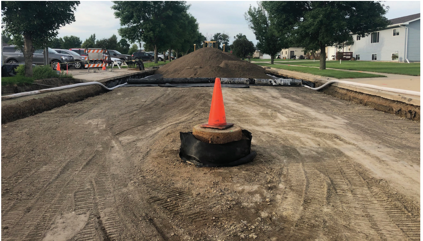
Work is progressing on State Street. About half of it has fabric, drain tile and gravel put down. Weather permitting, work will resume on Monday. (Photo by Paul Kosel)
