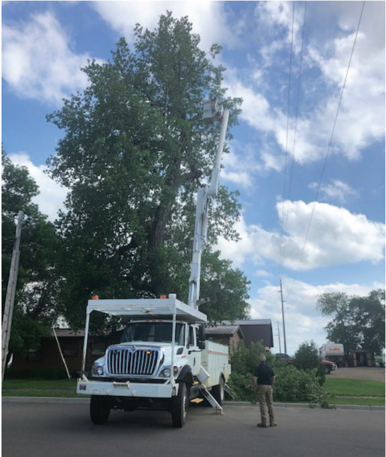
Treeline Tree Service trimmed the trees along the 69KV transmission line on the west side of town. The transmission line feeds the north substation. (Photo by Paul Kosel)
