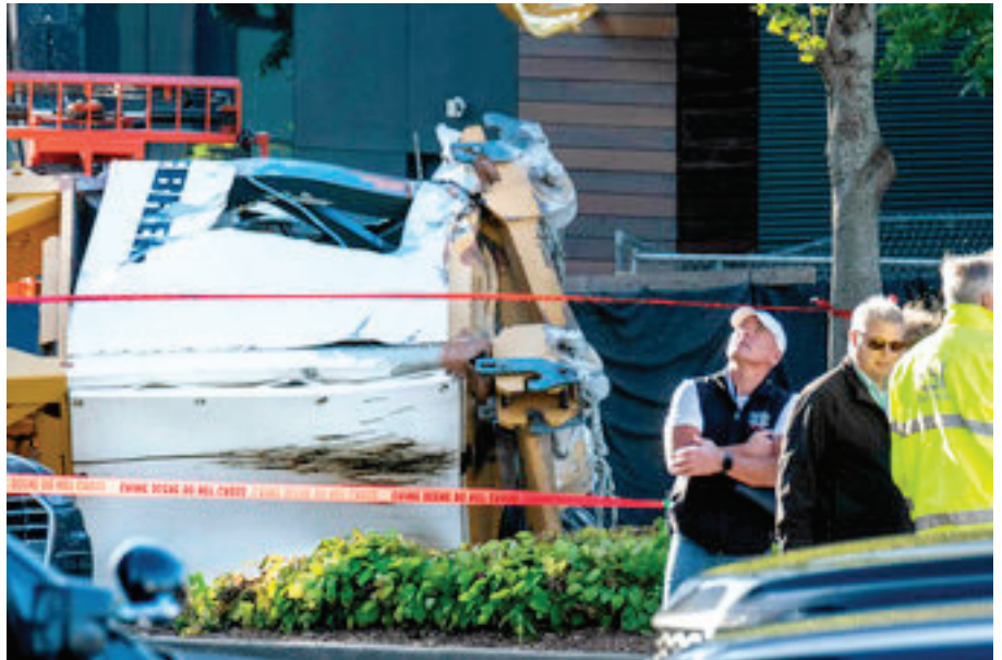
Police investigate the scene of a construction crane collapse near the intersection of Mercer Street and Fairview Avenue Saturday, April 27, 2019, in Seattle. Several people died and others were injured when a construction crane on the new Google Seattle campus collapsed Saturday, pinning cars underneath. (Dean Rutz/The Seattle Times via AP)
