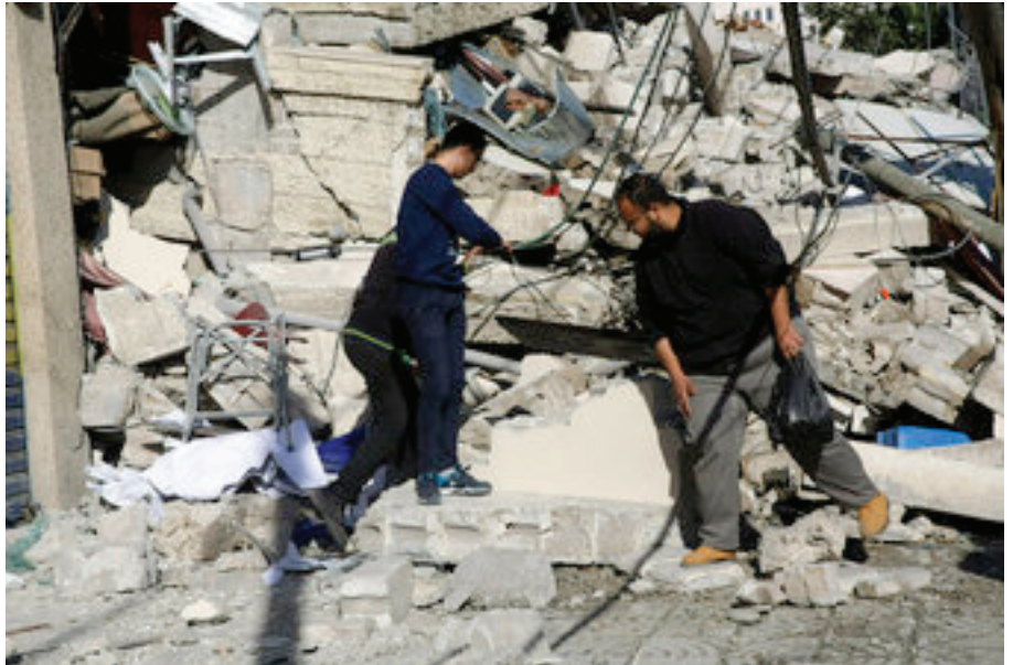
Palestinians inspect the damage of the destroyed multi-story building of Hamas-affiliated insurance company, in Gaza City, Tuesday, March 26, 2019. A tense quiet took hold Tuesday morning after a night of heavy fire as Israeli aircraft bombed targets across the Gaza Strip and Gaza militants fired rockets into Israel in what threatened to devolve into a major conflict two weeks before the Israeli election. (AP Photo/Adel Hana)
