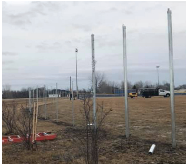
Work has been progressing on the new fence being installed at Falk Field at the Groton Baseball Complex. (Photo from Groton Baseball/Softball Foundation Facebook Page)
