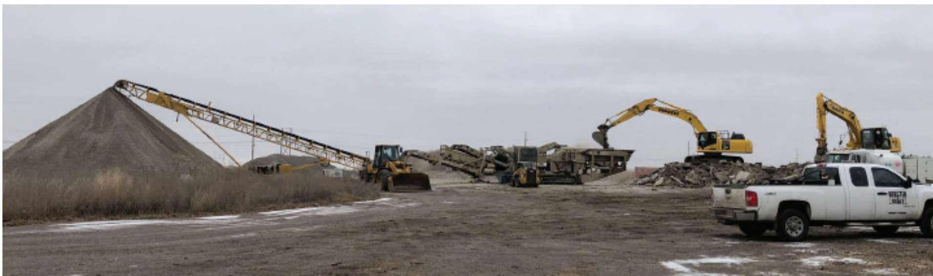
About 10 years of concrete accumulation is being ground up at the Groton rubble site. Webster Scale has been working at the site for the past week and work is expected to be completed by the end of this week. (Photo by Paul Kosel)
