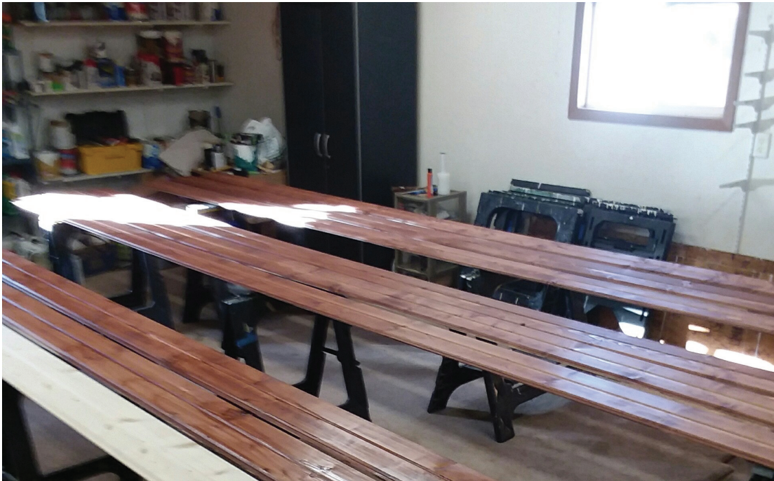
Ceiling boards and rafters are being stained in the Final Finish workshop of Shirlee Briggs to match the original boards in the interior of the church. (Photo by Betty Breck)
