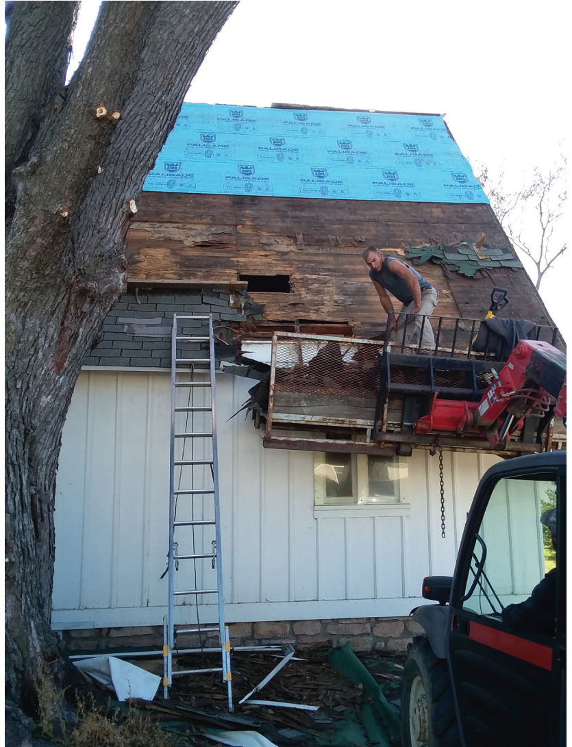
Blocker Construction started tearing off the old roof of Groton's Historic Trinity Church on Monday, and discovered a big hole under the old asphalt shingles on the North side. The new steel shingles will closely resemble the original 1884 wooden shingles. (Photo by Betty Breck)
