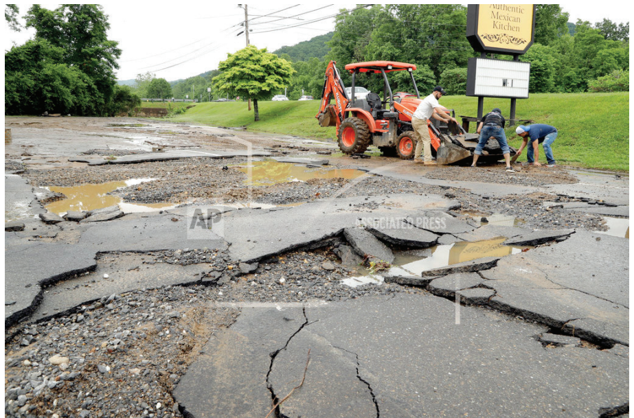
Workers clear debris from a parking lot washed out at a restaurant in Black Mountain, N.C., Wednesday, May 30, 2018 after heavy rains from the fringes of Subtropical Storm Alberto caused widespread flooding Tuesday evening. (AP Photo/Chuck Burton)
