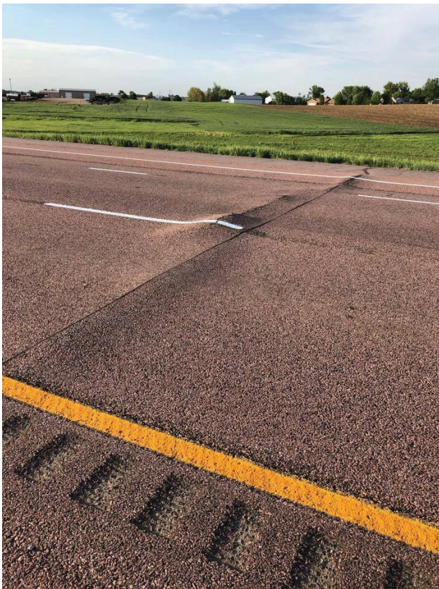
South Dakota DOT was called to Interstate 90 near Humboldt SD to fix this.
