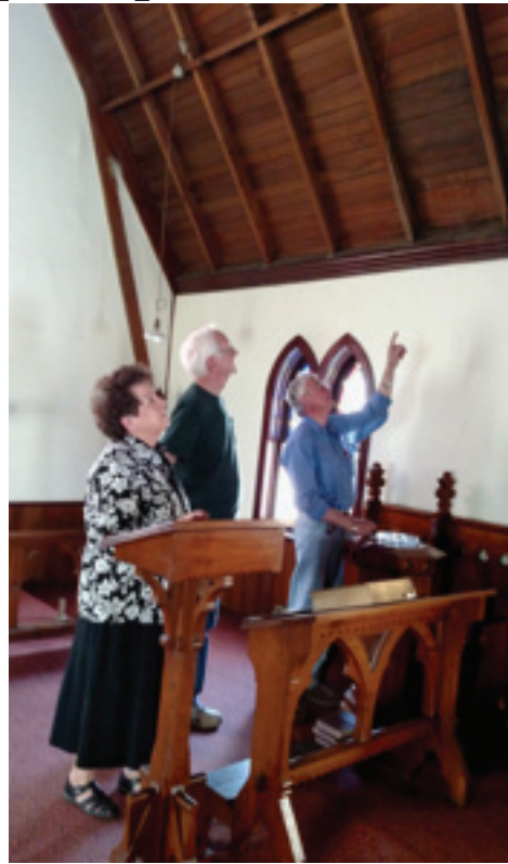
GCHS President "Topper" Tastad points to ceiling boards tacked over damaged roofing boards. (Courtesy Photo)
