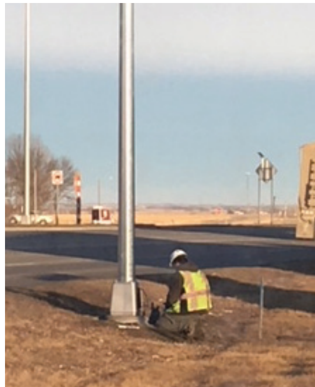
A worker from Muth Electric worked on a few of the street lights along US12 in Groton yesterday. There were a few that were not working and there is yet one more pole that needs to be installed.
