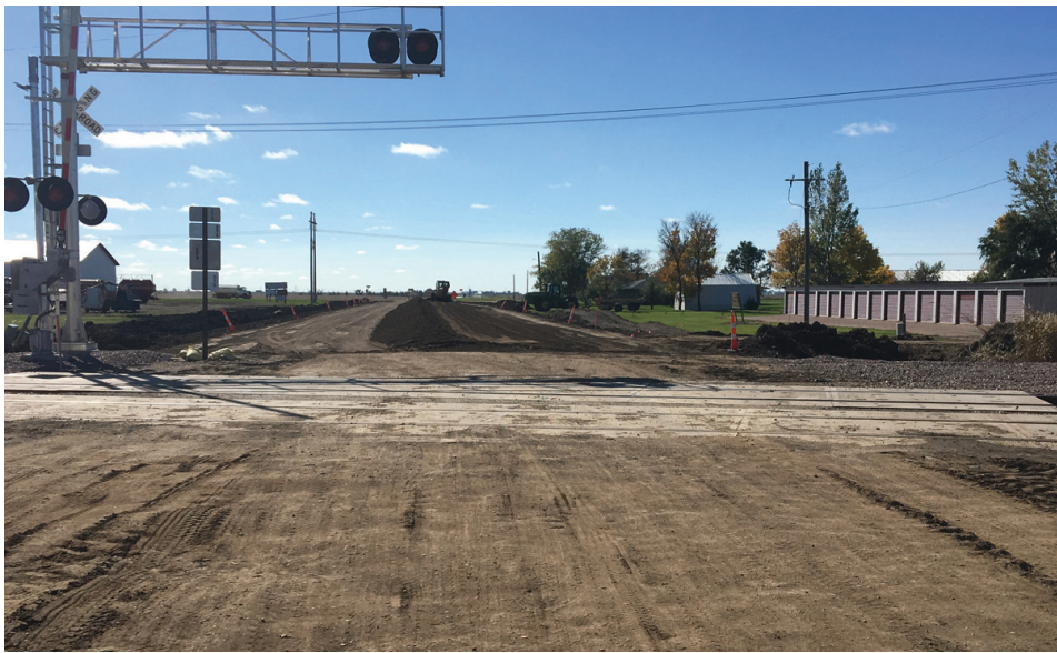
The final layer of base was put down in the Phase 6 part of the project on Thursday. (Photo by Paul Kosel)
