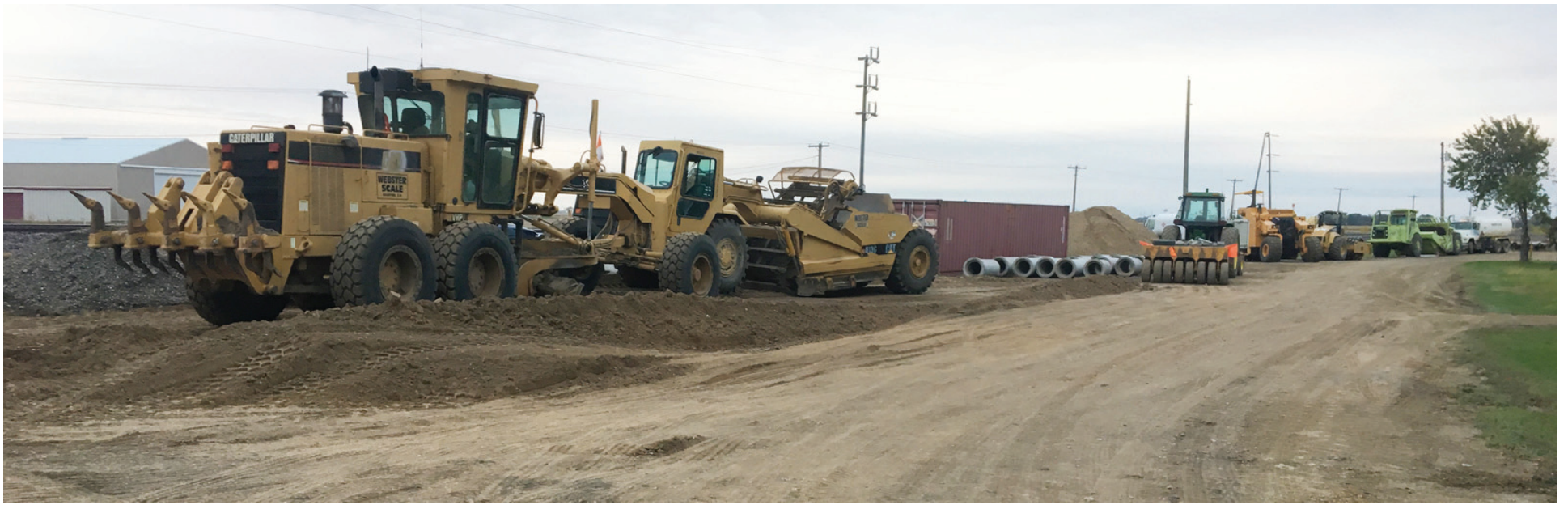
There is a lot of heavy duty equipment ready for action on the Phase 6 part of the SD37 project. The equipment has been on the city property just south of the railroad tracks. (Photo by Paul Kosel)
