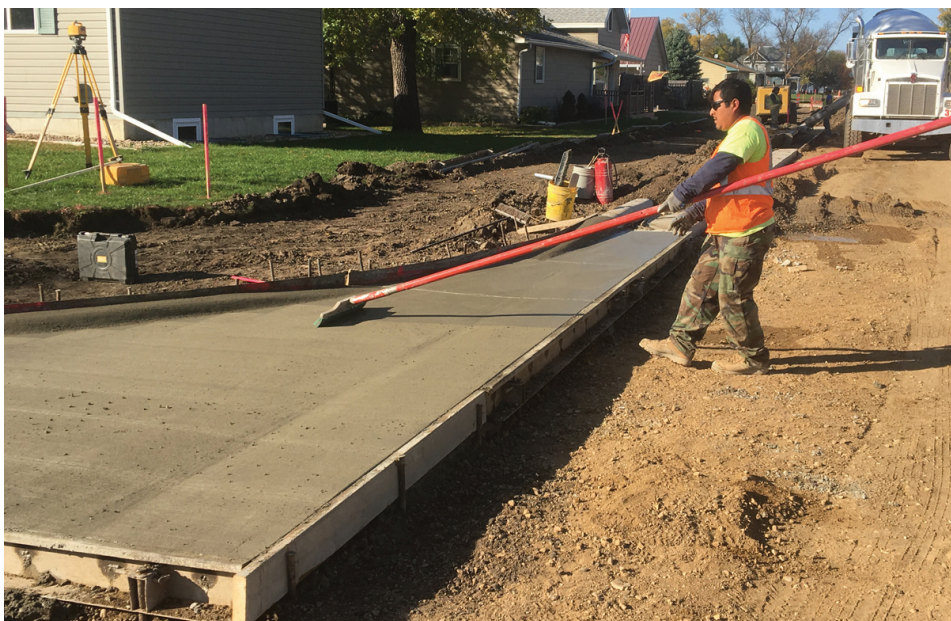
Pablo Xolo of Wright and Sudlow is putting the finishing touches on the freshly poured concrete. (Photo by Paul Kosel)
