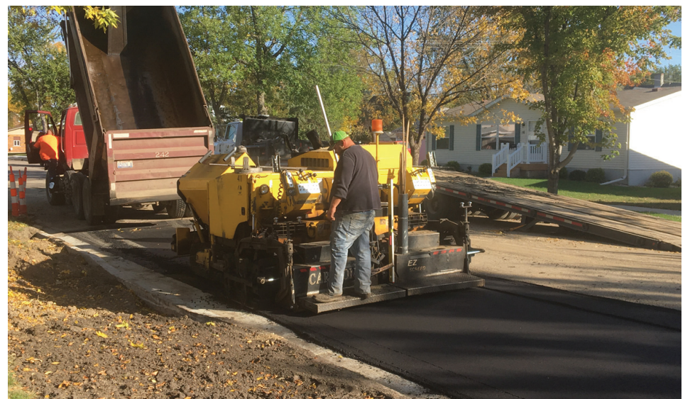
Lien Transportation was working on the Fourth Avenue part of the project. Part of the road had to be removed to lay new storm sewer pipe. The final layer of asphalt is being laid down in this photo. They will be doing more asphalt work on SD37 next week. (Photo by Paul Kosel)
