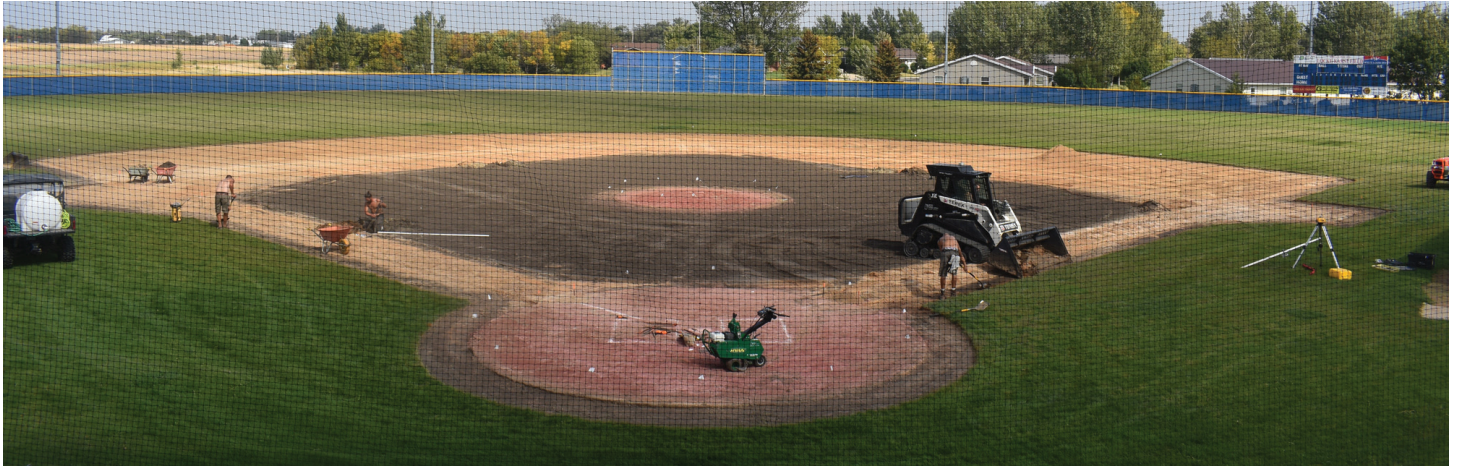
Locke-Karst Field is getting a new infield this year. Weber Landscaping has removed the sod and will be putting a new sod down next week. (Photo by Paul Kosel)
