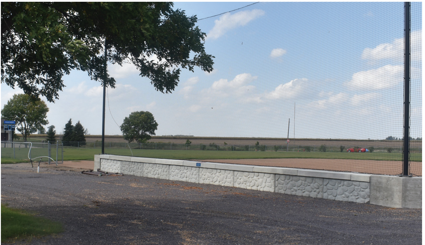
The dugouts on the smaller fields at the Groton Baseball Complex have been removed with new ones to be installed for the next season. (Photo by Paul Kosel)
