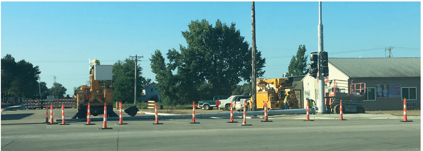
The Muth Electric crew was getting ready to lift one of the arms for the new signal lights at US12 and SD37 on Wednesday.
