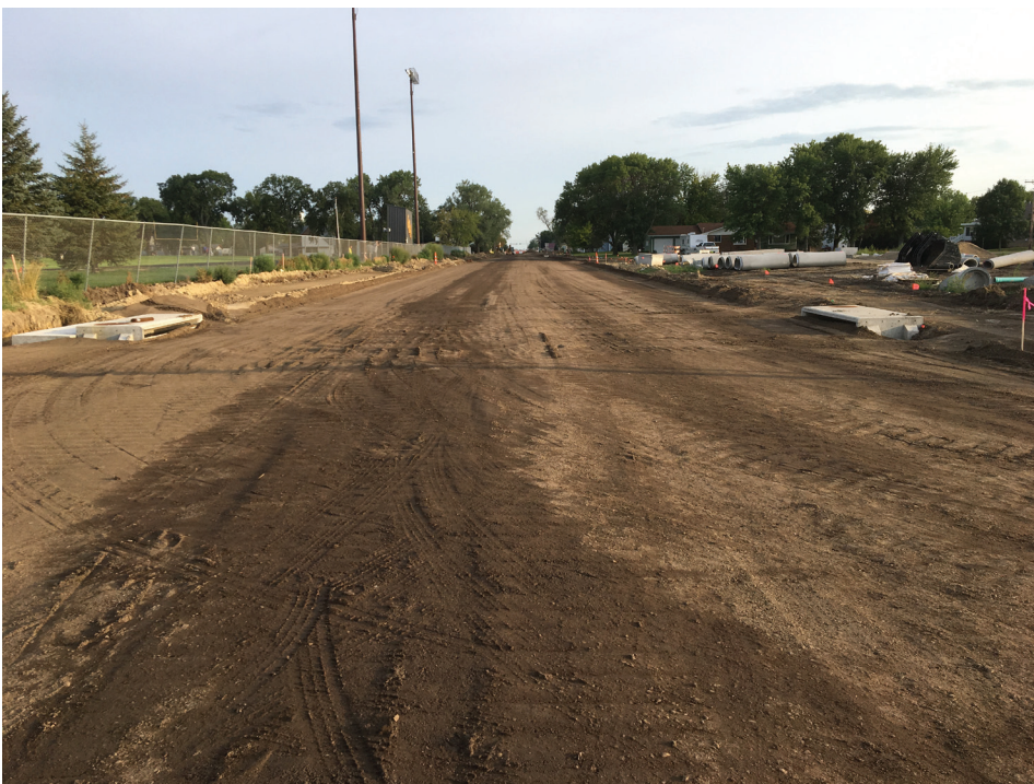
Even the road is starting to take shape on SD37. This view is looking south at Seventh Avenue.
