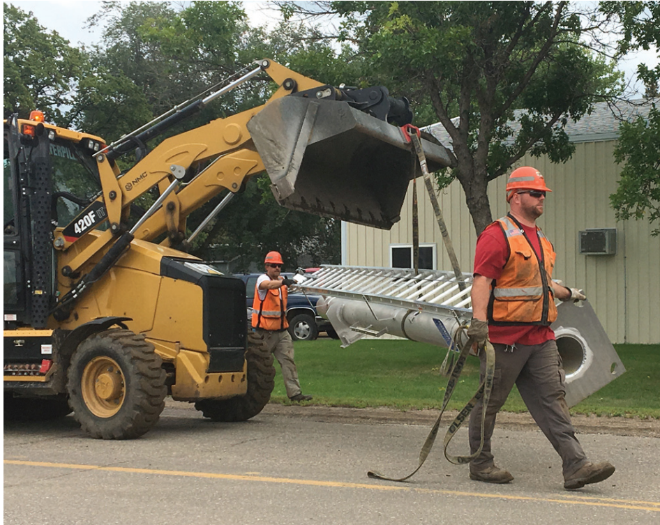
Burlington-Northern Railroad workers were guiding a new crossing to its resting place. The railroad cross on the south edge of Groton is being replaced as part of the highway project.
