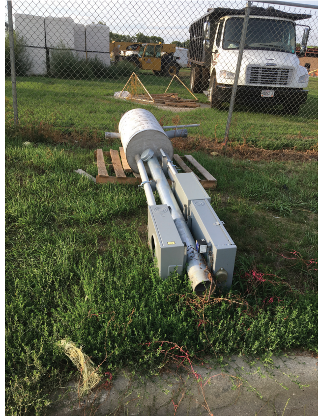
This is the electrical hookup for the new lights to be installed on SD37 in Groton.
