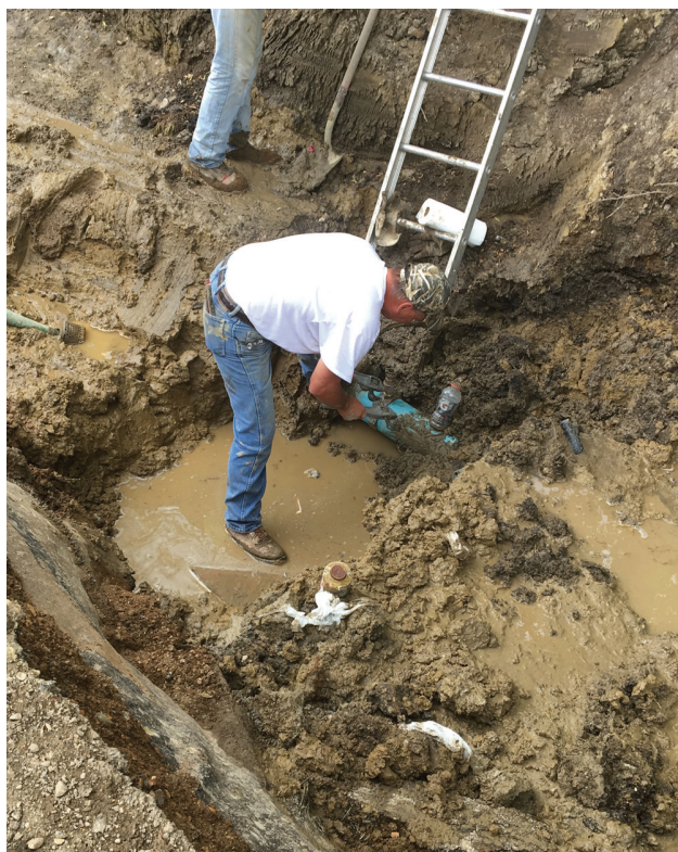
Terry Herron was fixing a water leak caused by Webster Scale, Inc. on Monday. The water service line feeding Mary Larson's home was accidentally pulled up on Monday.
