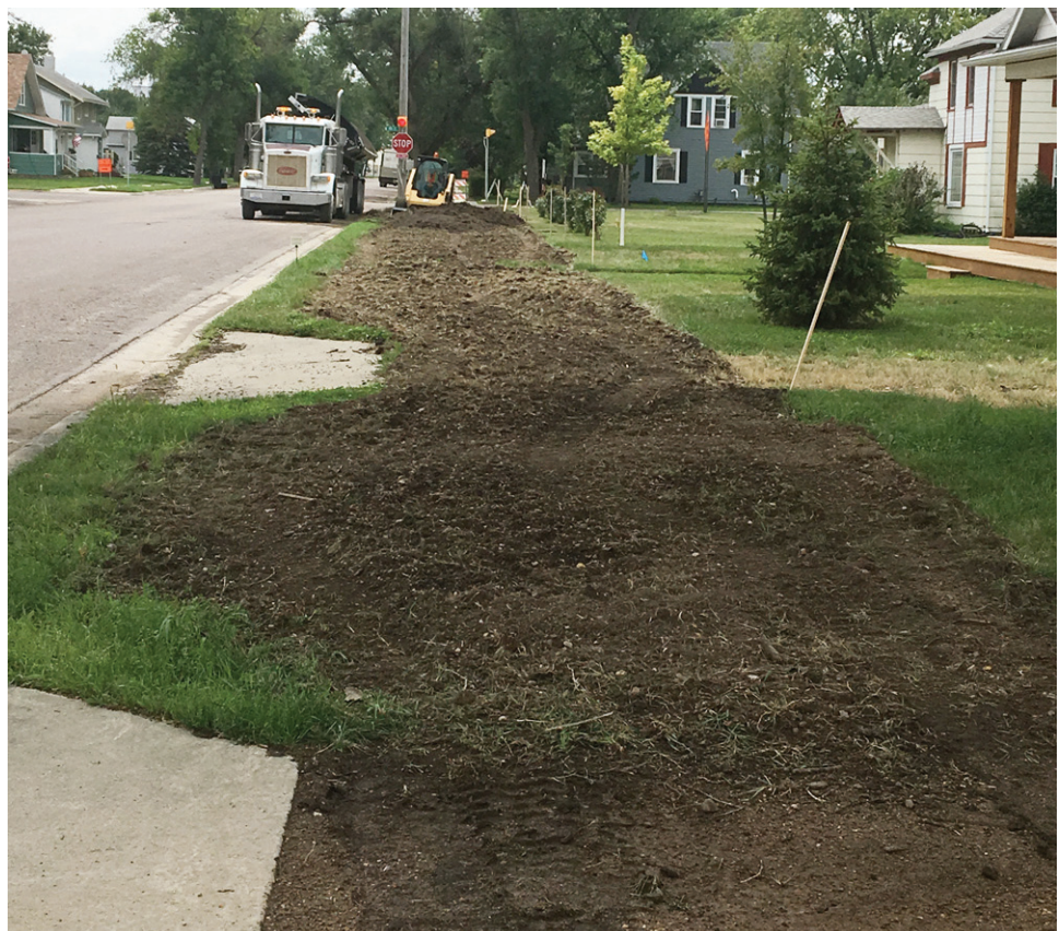
Work is beginning on the Safe Route to School sidewalk. It will run on the west side of First Street from Fourth Avenue to Fifth Avenue. Then on the north side of Fifth Avenue from First Street to Lincoln Street.
